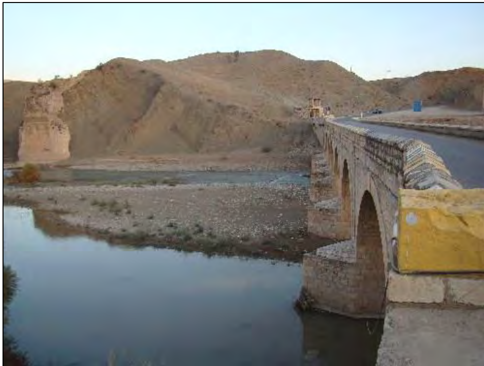
Lorestan, Karkheh River at Kashgan Bridge (Kashgan Bridge, Iran1, CC BY 3.0, Kazem Fattahi).
